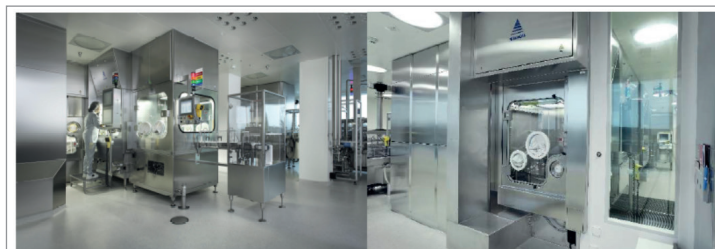
Figure 2. Isolator for loading and unloading a freeze dryer.
